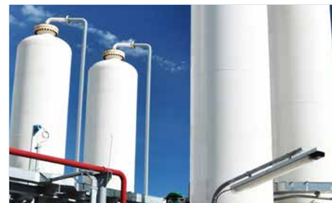
Storage of technical gases
